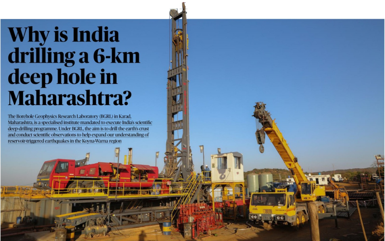
DEEP DIVE: At the deep drilling site in Koyna region, Maharashtra, the towering drilling rig is seen surrounded by associated equipment, an onsite mud logging unit, gas analysis lab, and a geological studies lab. MOTES-BGRL
